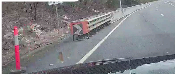
Sudden change in temporary barrier in roadworks
